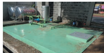
Effluent treatment facility
