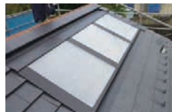
Energy generation system using roof integrated high-efficiency vacuum thermal energy
