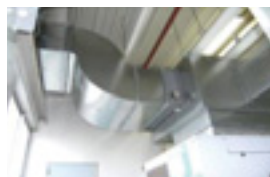
An exhaust duct used for heating as well
