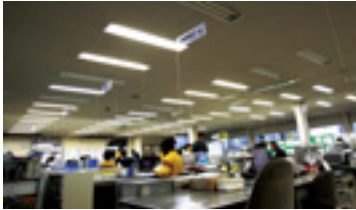
Ceiling lights can be individually switched on and off
