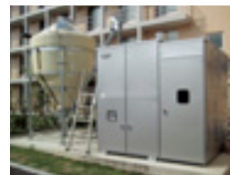
a wood pellet fired Aroace chiller/heater in use in the Y-TOWN
