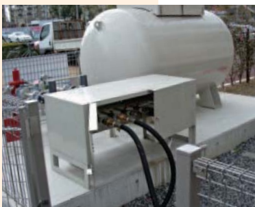
Gas storage tanks for use by local residents in the event of an emergency
