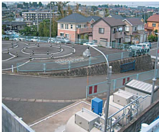
Green Station (bottom right) installed at a driving school
