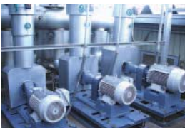
Secondary chiller-heater pumps
