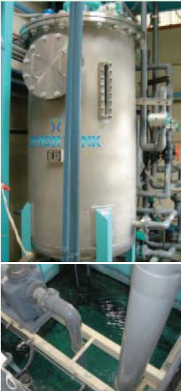
Sand filtration system at the non-industrial sewage treatment facility
