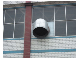
Exhaust duct before improvement
