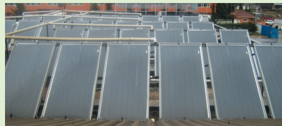
Solar panels installed on the roof of the Kuzuluk Factory
