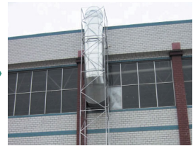
Exhaust duct after improvement
