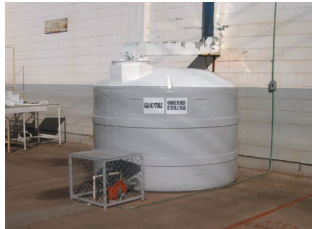
Rainwater-collection tank installed on the factory grounds
