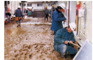
Yazaki gas equipment authorized dealers performed construction of LPG facilities for temporary housing
