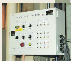
Device to control the number of air compressors
