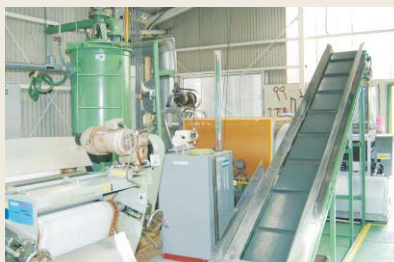
Sludge to fertilizer conversion plant built inside the factory
