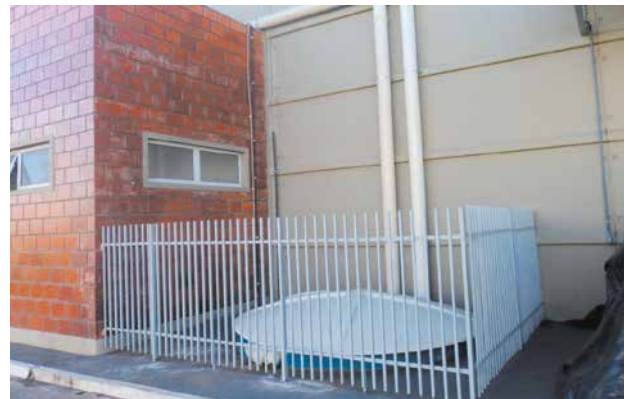
A rainwater tank installed at YBL (Brazil)
