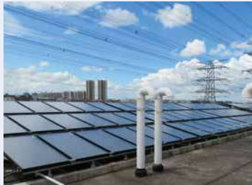
Solar panels installed on the company dormitory
