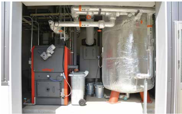
Biomass chip boiler constructed for Fujiyama Village
