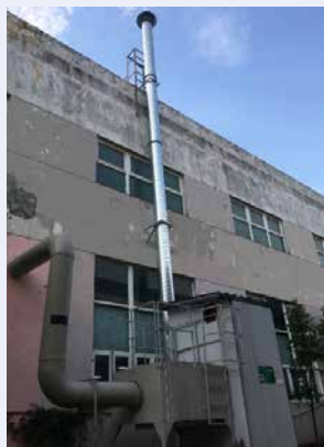
VOC (exhaust gas) processing facility
