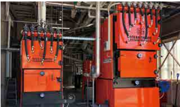
District heat supply biomass boiler
