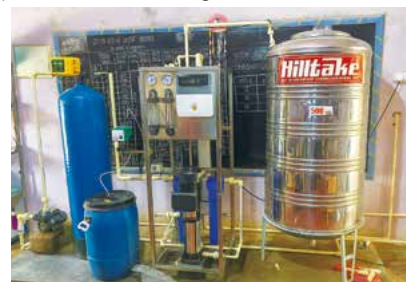
Treatment tank and filtration system
