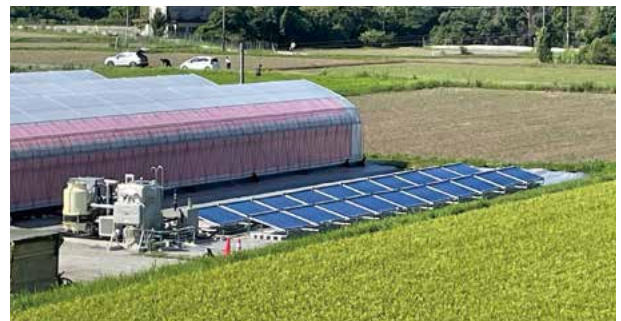
Agricultural greenhouse for tomato cultivation at POMONA FARM, utilizing the solar cooling air-conditioning system product
