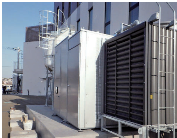
Bio-Aroace wood pellet-fueled absorption chiller-heater installed at Kasakakenishi Elementary School in Midori City (Midori City, Gunma Prefecture)
